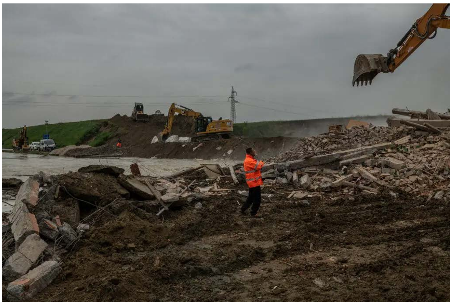
Excavators worked on the banks of the Santerno River to build a dike and tear down a home that had been severely damaged by the floods. Elisabetta Zavoli for The New York Times
